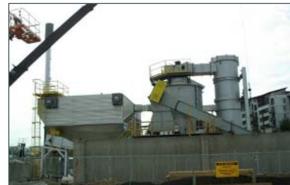
Dockside Green Gasification Plant
